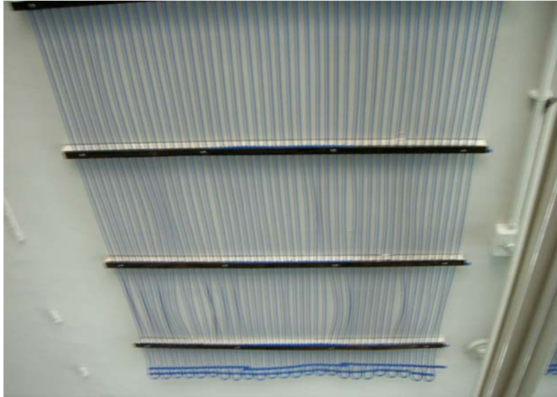
Fig.7 Ceiling capillary cold radiation system
