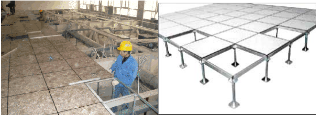
Fig.5 Overhead moving floor used in the building
